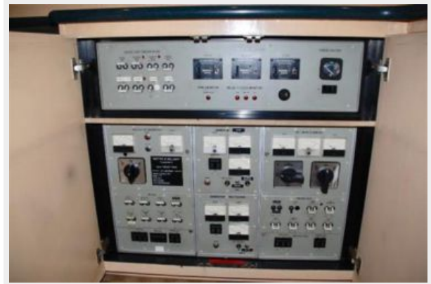
Electric Distribution Panel
