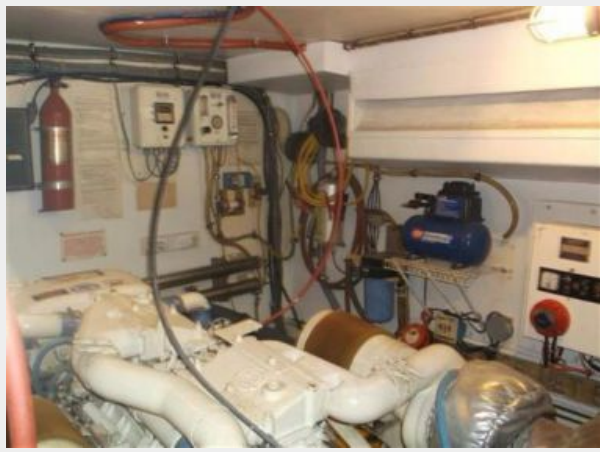
61' Hatteras - Engine Room 2
