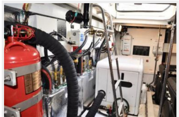
Engine Room Side View
