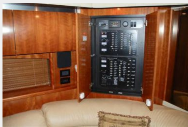
Power Distribution Panel
