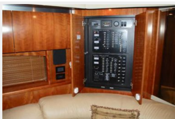
Power Distribution Panel
