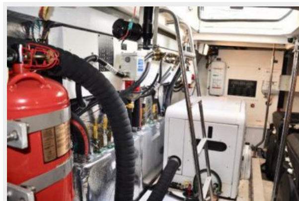
Engine Room Side View
