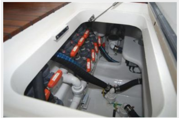
Viking 55 Convertible - Pump Controls
