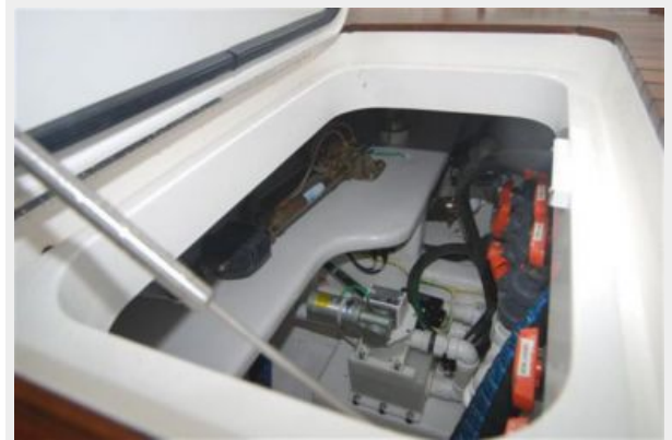
Viking 55 Convertible - Pump Controls
