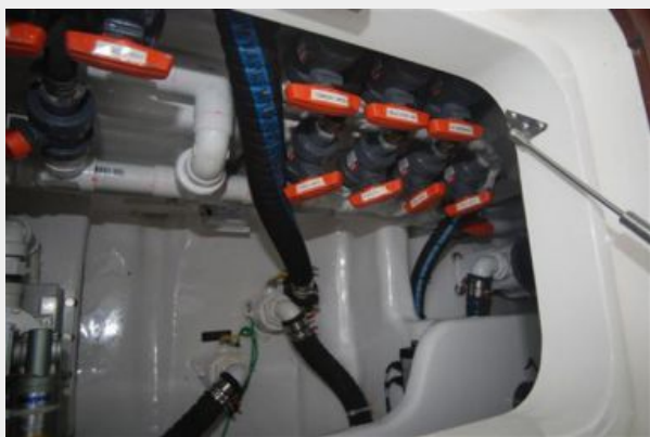
Viking 55 Convertible - Pump Controls
