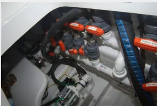
Viking 55 Convertible - Pump Controls
