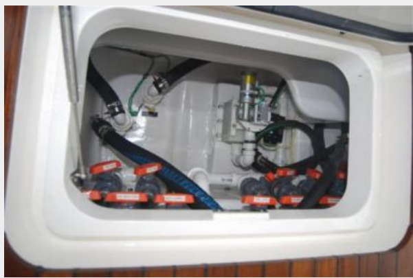
Viking 55 Convertible - Pump Controls
