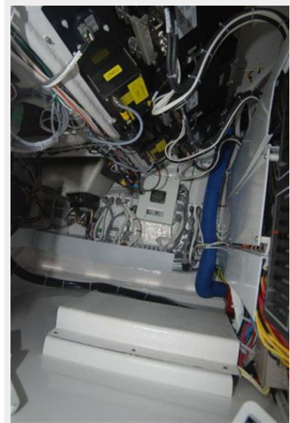
Viking 55 Convertible - Pump Controls
