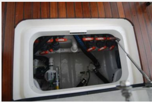
Viking 55 Convertible - Pump Controls
