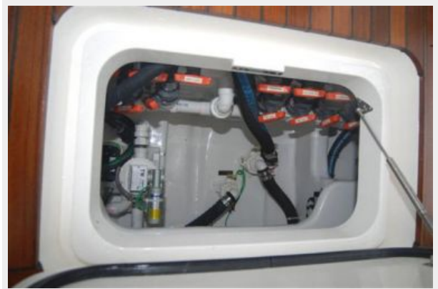
Viking 55 Convertible - Pump Controls
