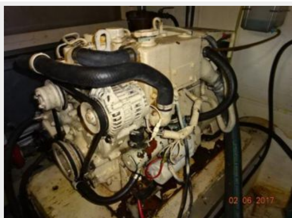
1979 Grand Banks Classic 42 Kohler Generator
