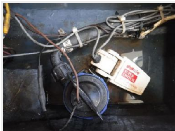
Bilge pump and switch
