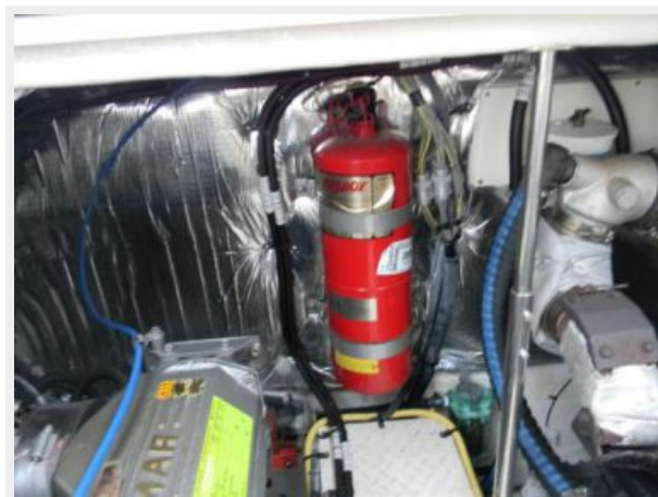
Automatic Fire Extinguisher System
