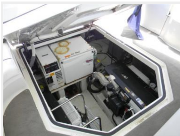
Engine Room Access
