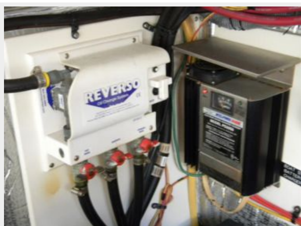
Oil Exchanger System
