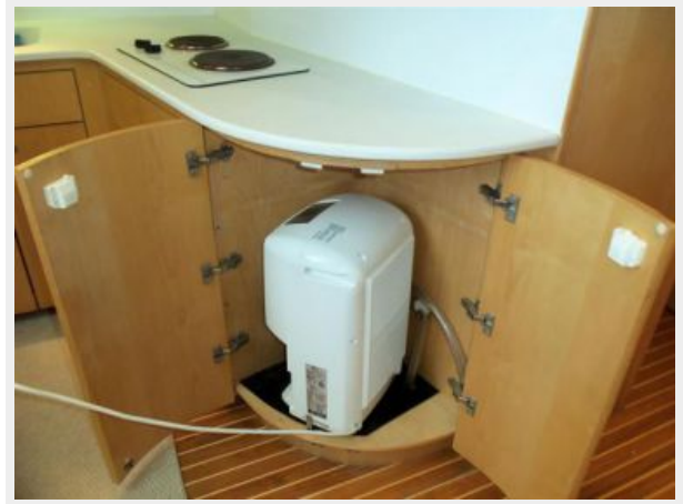
Permanently Installed Dehumidifier
