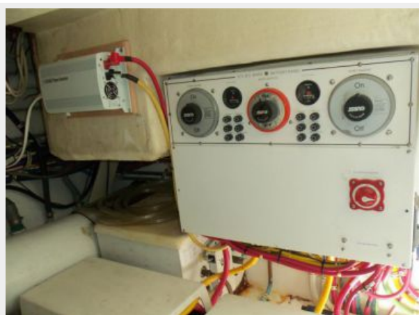
Engine Room Aft
