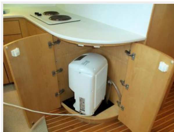
Permanently Installed Dehumidifier
