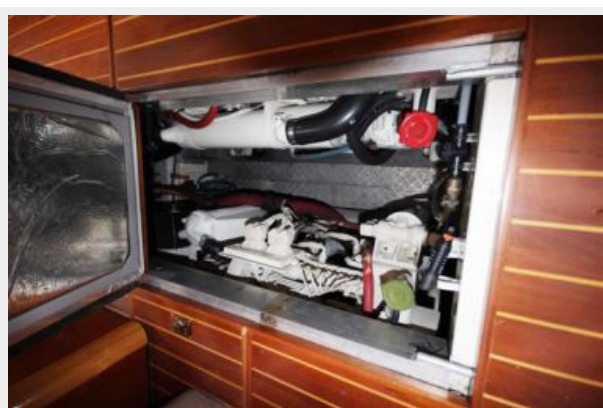
Clean Engine Room
