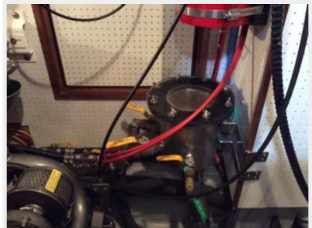
Engine Compartment Raw Water Manifold
