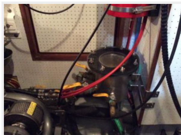
Engine Compartment Raw Water Manifold
