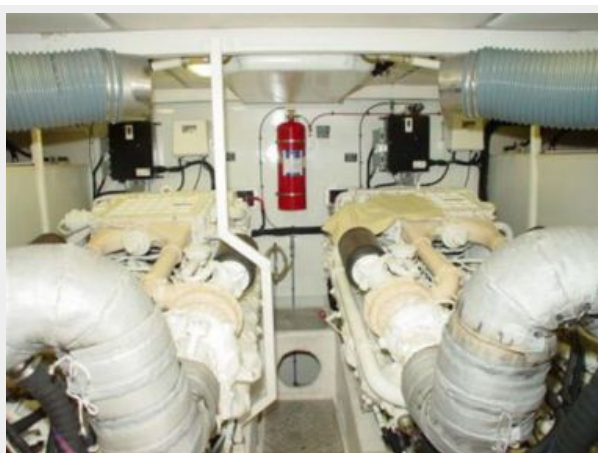
65' Princess Viking - Engine Room
