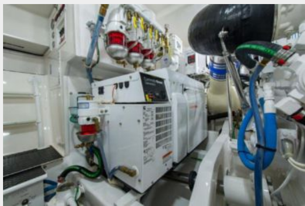
Engine Room Port
