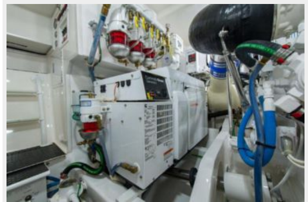
Engine Room Port
