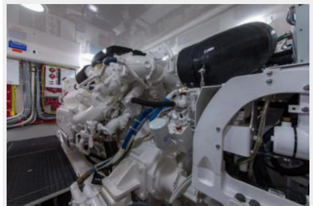
Engine Room Starboard
