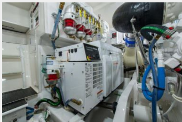
Engine Room Port
