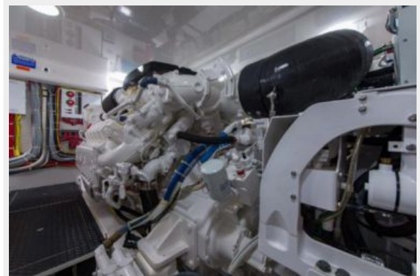
Engine Room Starboard
