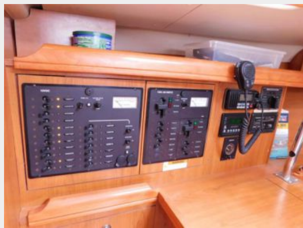
38' Hunter electrical panel
