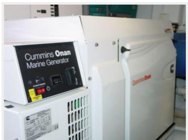
Electrical System / Equipment - Generator
