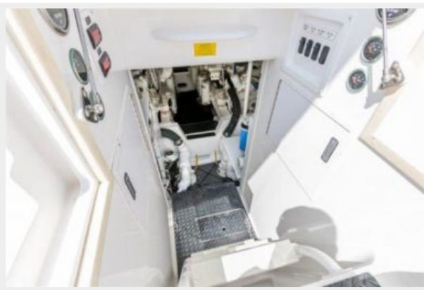
Engine & Mechanical Equipment 1
