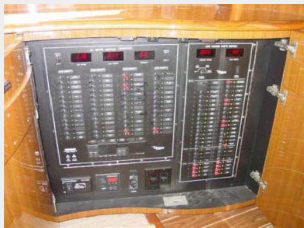
Salon 6 - Electrical Panel
