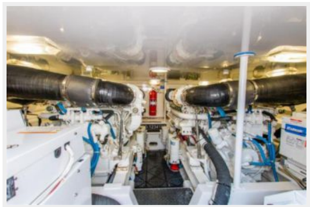
Engine & Mechanical Equipment 2
