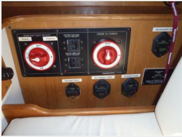
Electrical Control Panel
