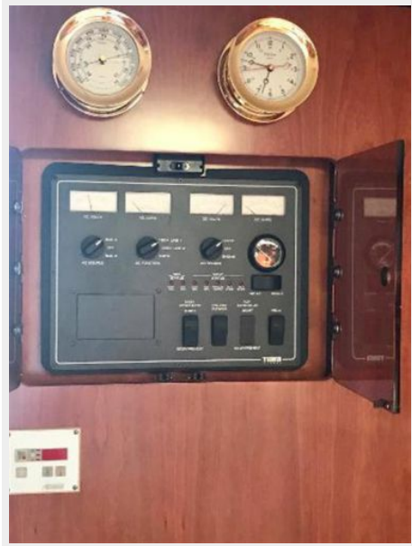
Shore Power/ Genset Panel
