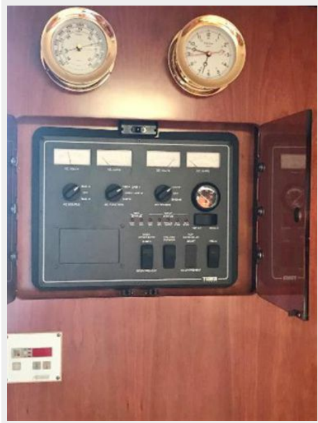
Shore Power/ Genset Panel
