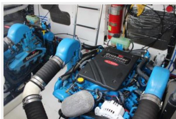
36 Tiara Sovran Engine Room
