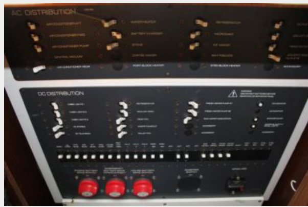
36 Tiara Sovran Control Panel
