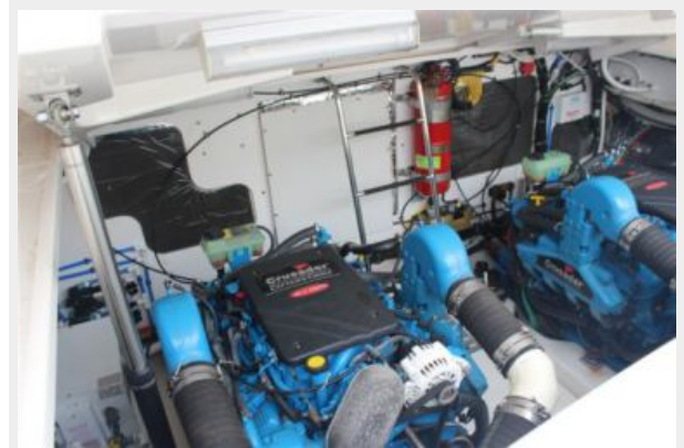
36 Tiara Sovran Engine Room
