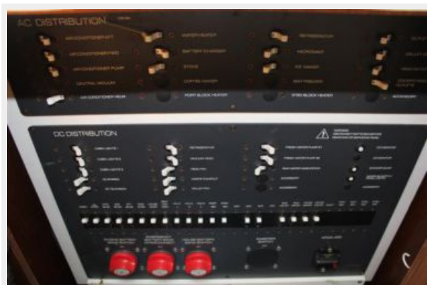
36 Tiara Sovran Control Panel
