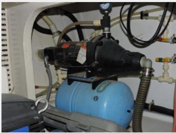
Engine Room - Water Pump
