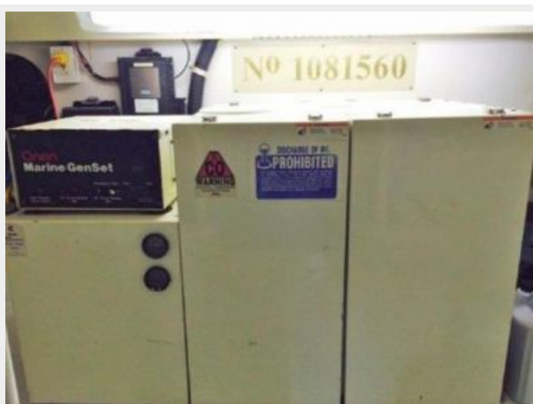
Engine Room - Generator
