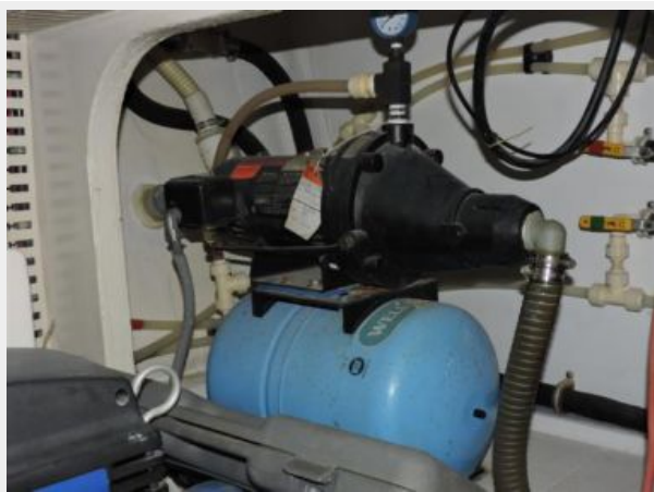
Engine Room - Water Pump
