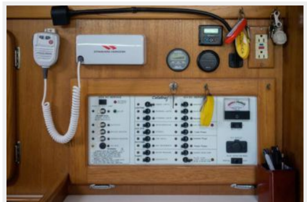
Chinook19 Electrical panel
