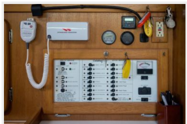
Chinook19 Electrical panel
