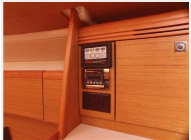
Galley A/C Control and Propane Control
