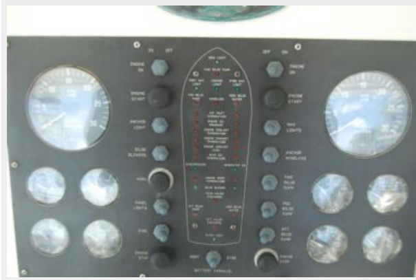
Helm Control Panel.JPG
