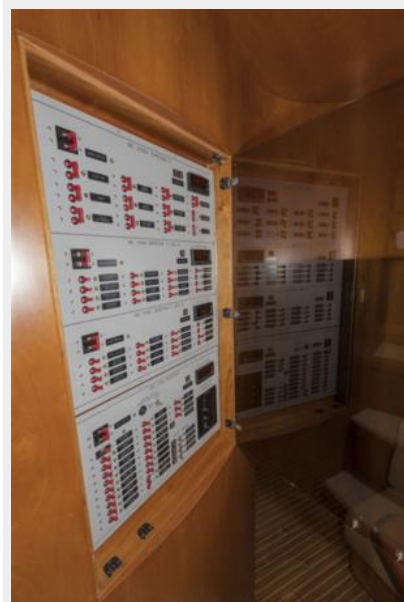
Crew Electrical Panel
