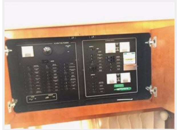
Circuit breakers on std side of salon.
