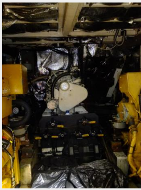
Grand Banks 42 - Engine Room Generator
