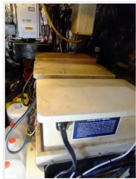
Grand Banks 42 - Engine Room Battery Bank
