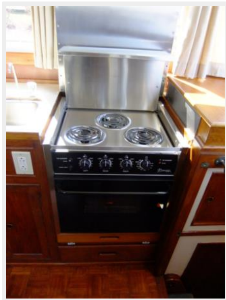
Grand Banks 42 - Galley Electric Stove Top & Oven
