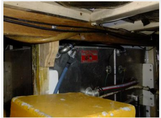
Grand Banks 42 - Engine Room New Fuel Tank STBD Side
