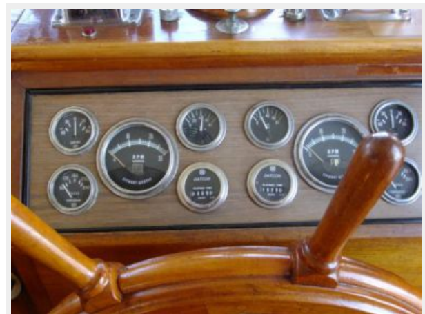
Grand Banks 42 - Helm Station Dual Engine Gauges.
