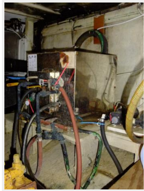
Grand Banks 42 - Engine Room HW Heater
