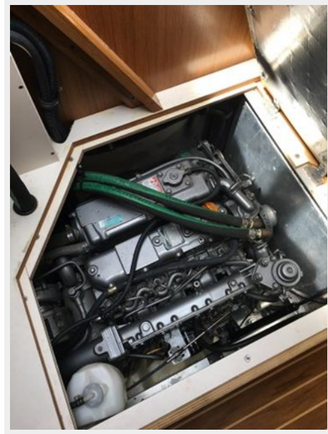
2004 Catalina 470 - Clean engine space
