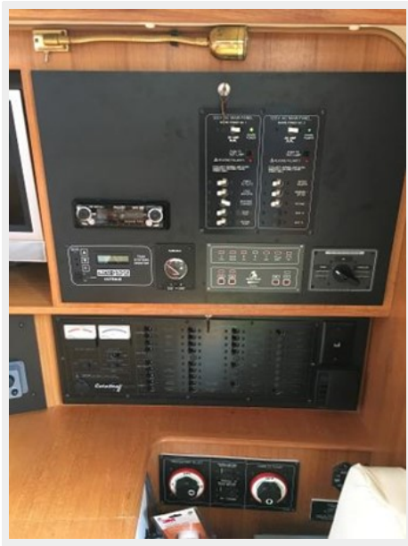
2004 Catalina 470 - Electrical distribution panel/ Nav station
