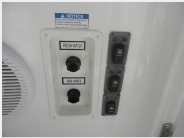
Fresh and raw water wash down
