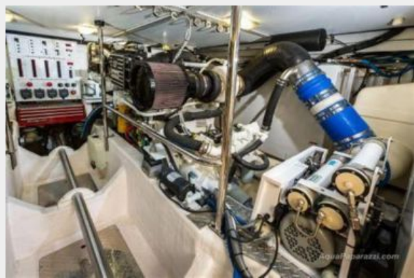
52 Sabre Engine Room
