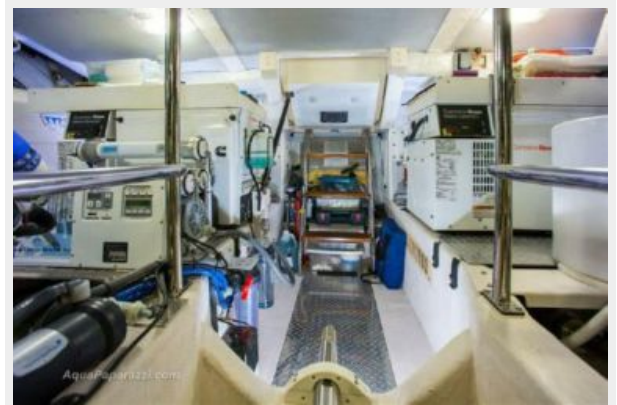
52 Sabre Engine Room
