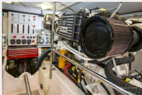
52 Sabre Engine Room
