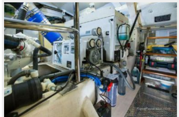
52 Sabre Engine Room
