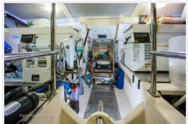
52 Sabre Engine Room
