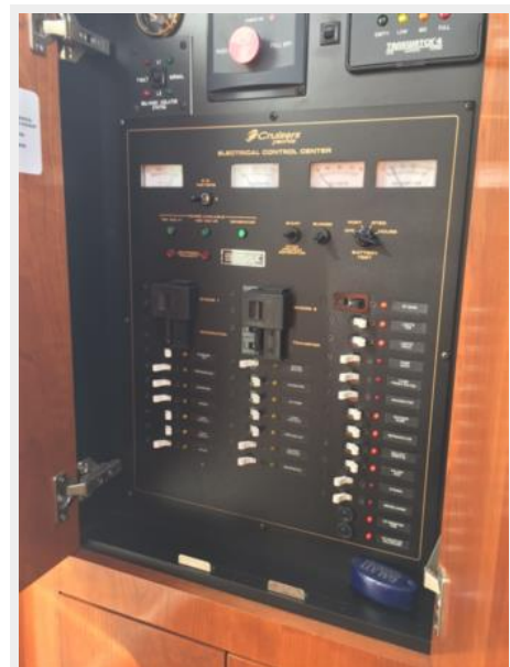
Main Distribution Panel
