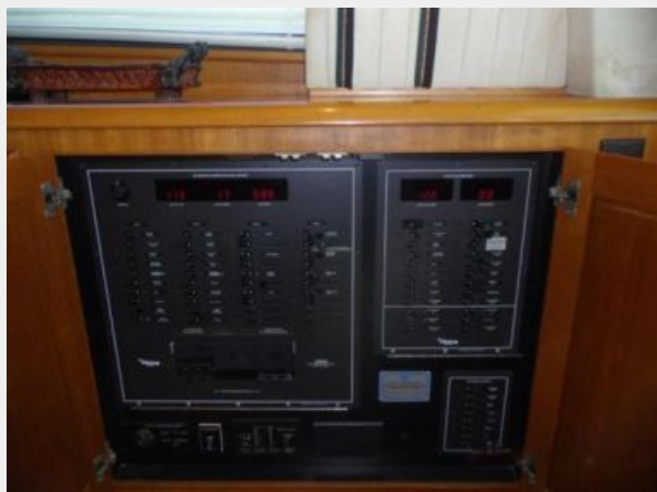
Electrical System / Equipment 1 - Electrical Panel
