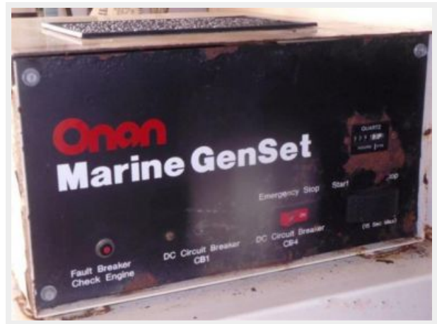
Electrical System / Equipment 2 - GenSet
