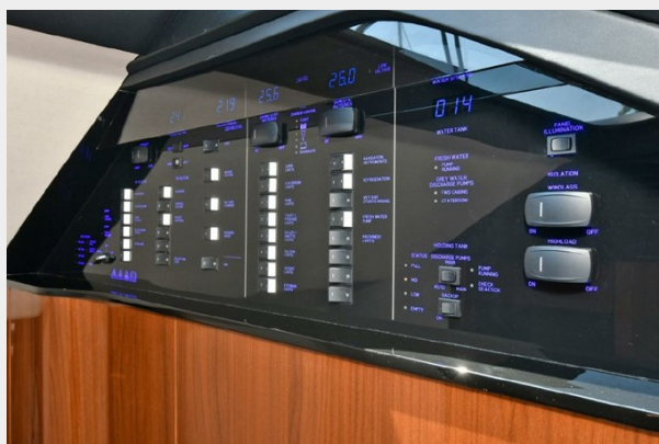
Salon Control Panel
