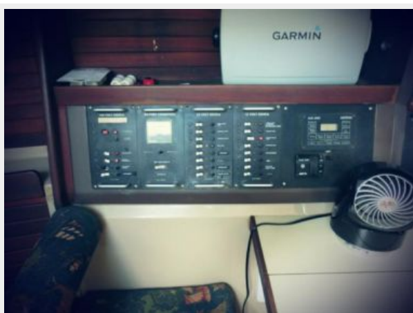
C & C 41 Electrical Panel
