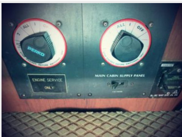
C & C 41 Battery Switches
