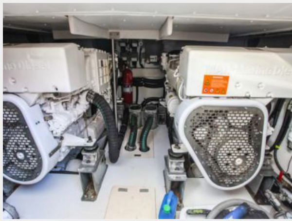
Engine Room Detail
