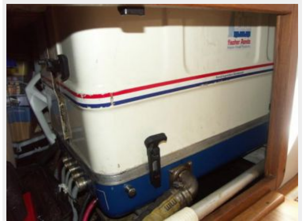
Panda Fisher Generator
