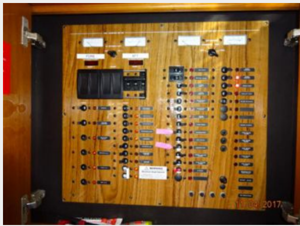
Moondance electrical panel 11-4-17
