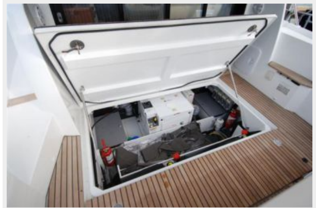
Cockpit access to generator and storage
