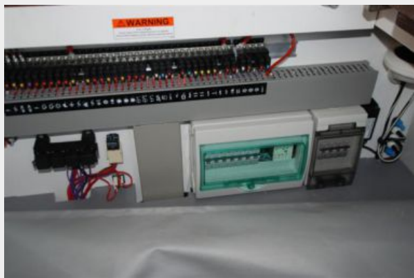
Electical breakers in Aft Storage
