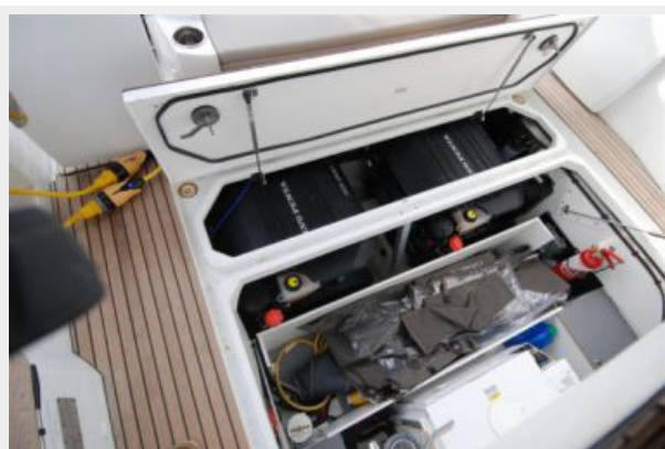
Cockpit access to generator, storage and engine compartment
