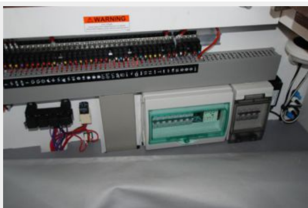
Electical breakers in Aft Storage
