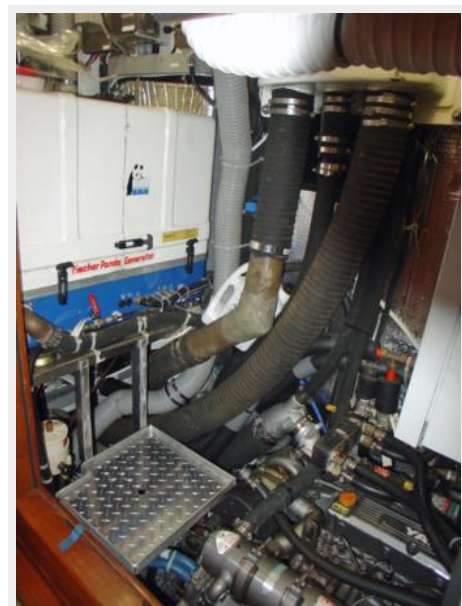
Engine Room, Aft
