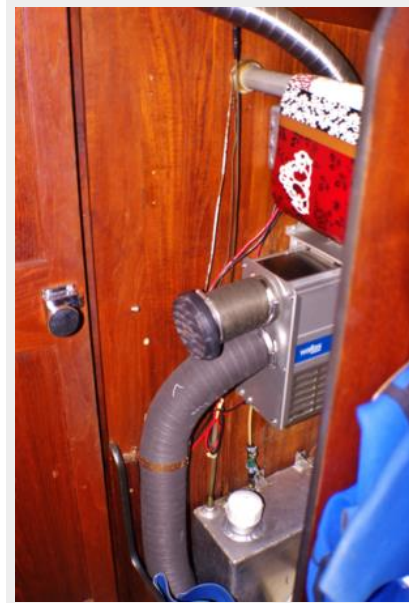
Forced air heater installation in the hanging locker
