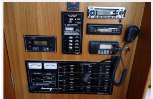
Nav Station Panel
